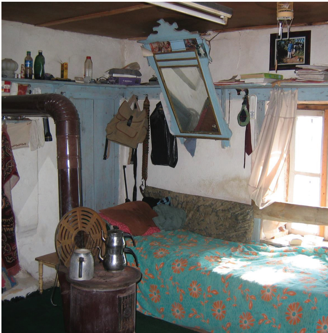
Figure 76. Biomass stove that is used in Sönmezer House
