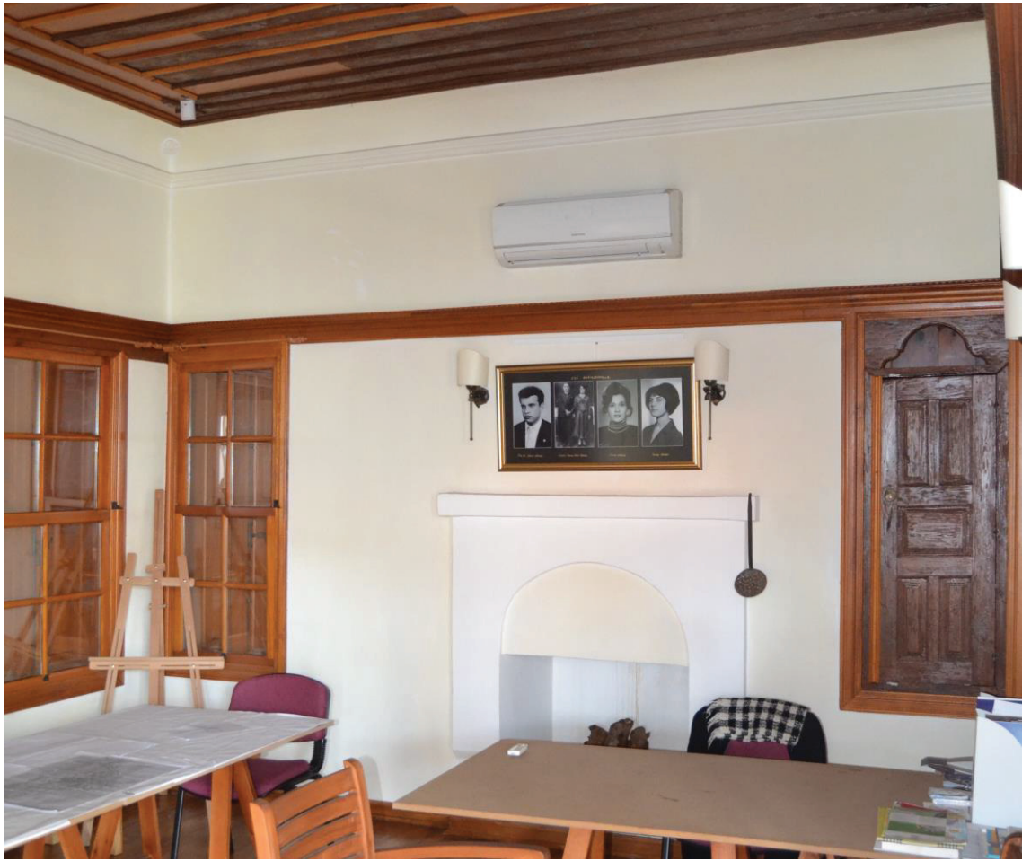
Figure 77. Air-conditioner that is used in Gürsel House
