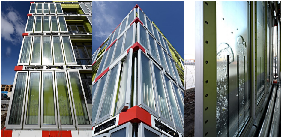
Figure 28. Algae House photo by Colt International, rotating louvers around a vertical axis to track sunlight, SSC GmbH, BIQ- AirLift-System bubbles rising in the SolarLeaf Louvers 31
