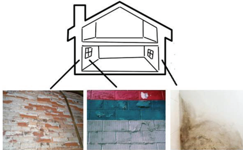
Figure 3. Damages are on the building wall due to moisture accumulation
