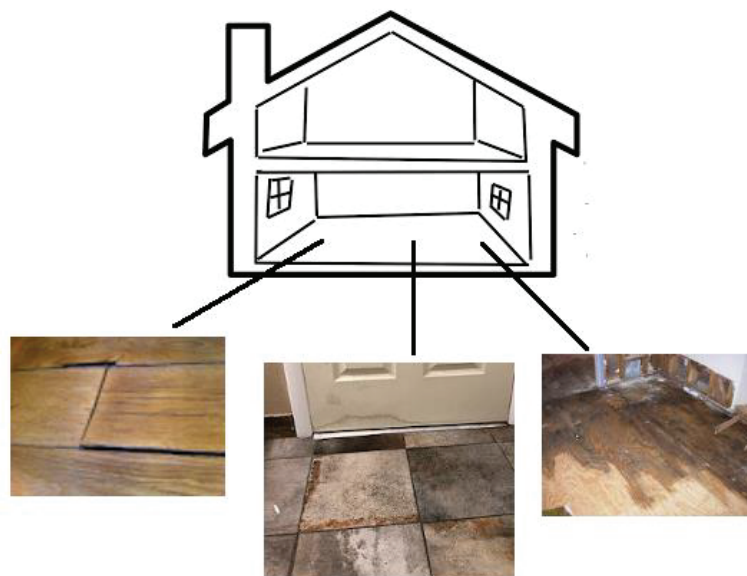
Figure 2. Damages on the building floor due to moisture accumulation
