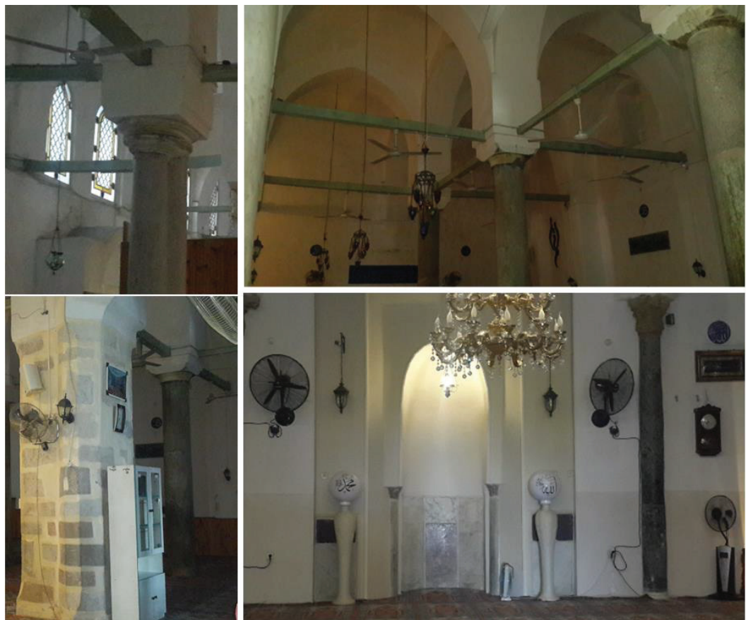
Figure 4.5. Fan locations in the prayer hall a) wall type fans, b) ceiling fans, c) portable fans
