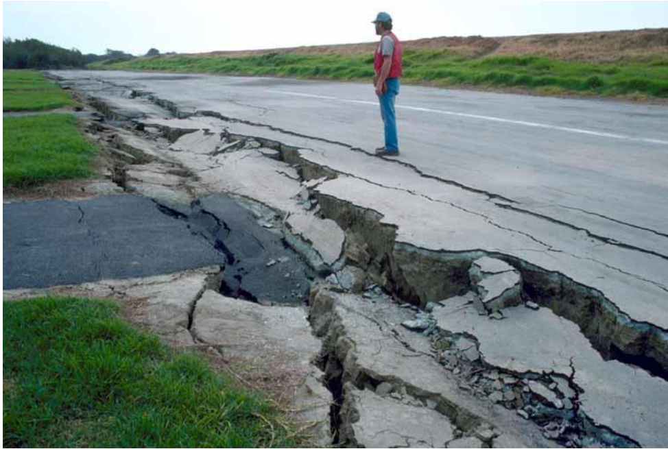
Figure 2.15. Lateral spreading (Source: wikipedia).
