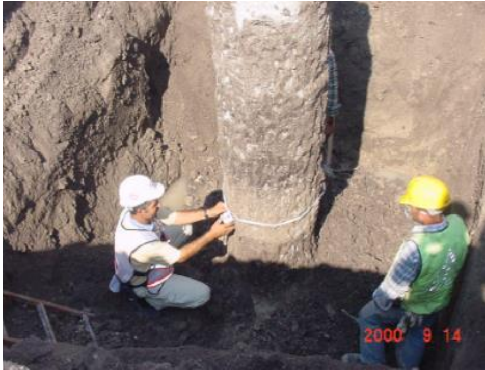
Figure 3.22. Investigation excavation and diameter control of jet grout column (Source: Gökalp and Düzceer 2000).
