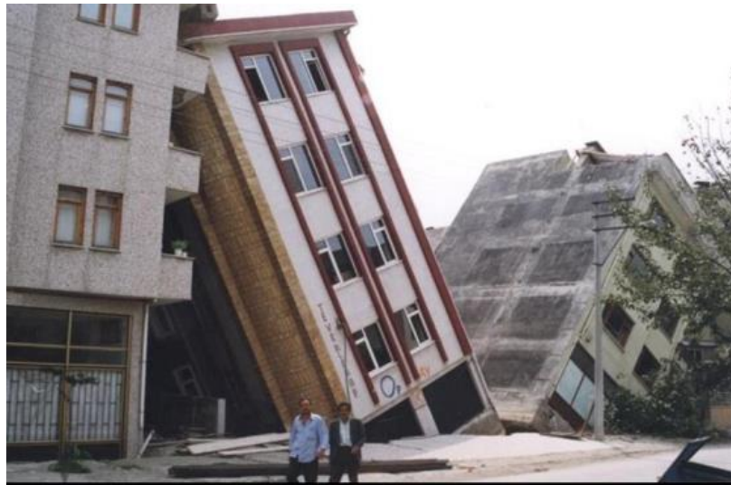
Figure 2.13. Major tilting of the buildings due to subsoil liquefaction (Source:Ada Pazarı 1999).
