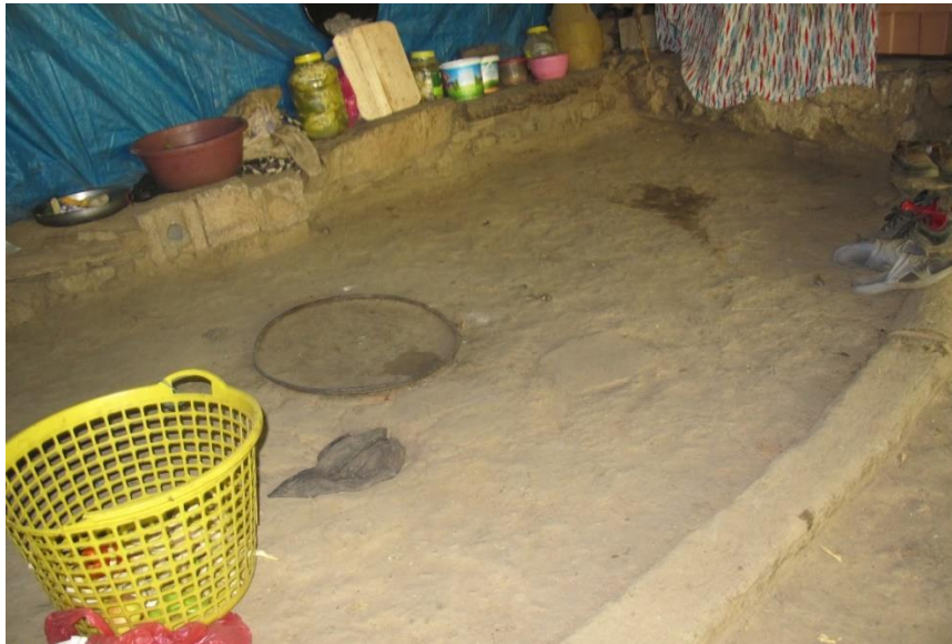
Figure 4.58. Level difference in the house of M&Z Bingöl (September 21, 2017).
