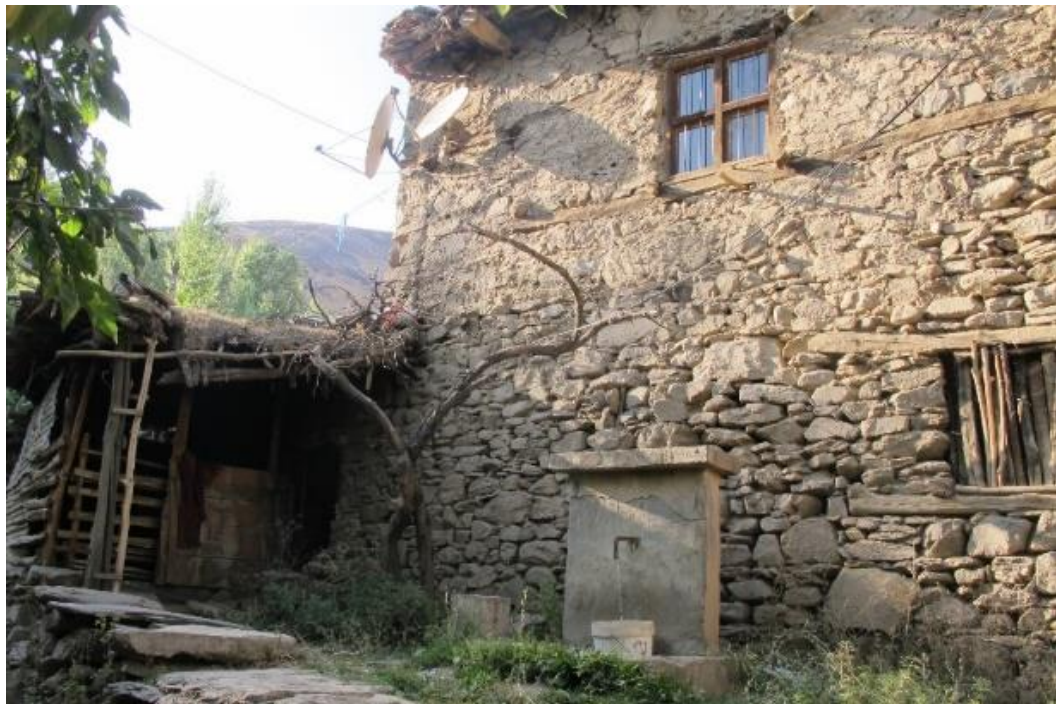
Figure 4.55. Distinguishable bonding of the upper storey (September 12, 2017).
