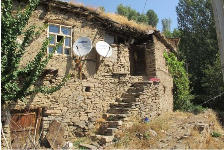
Figure 4.56. Distinguishable bonding of the upper storey (September 16, 2017).
