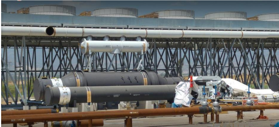
Figure 3.4. Air Cooler Condenser and Turbine-Generator
