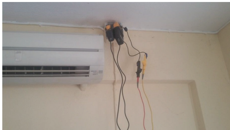
Figure 5.10. Power analyser to measure energy consumption of air-conditioner (Source: Extech, 2018)
