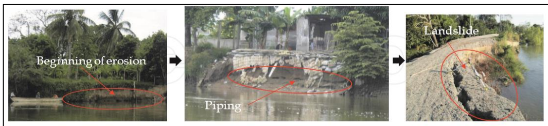
Figure 3.14 Evidences of instability in river embankments caused by erosion (Source: Jeanmonod and Rebecca 2018)
