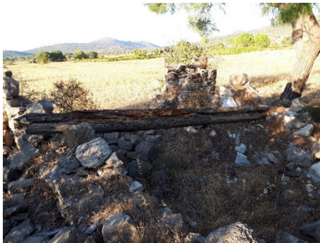
Dislocated main beam. September 24, 2017
