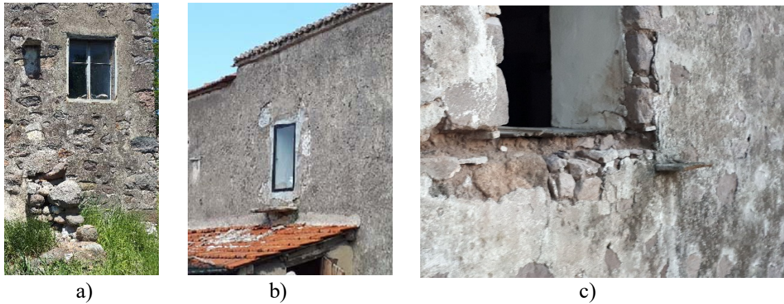
Figure 71. Exterior cantilever slate stones a) April 27, 2017. b) April 23, 2017. c) June 6, 2017.
