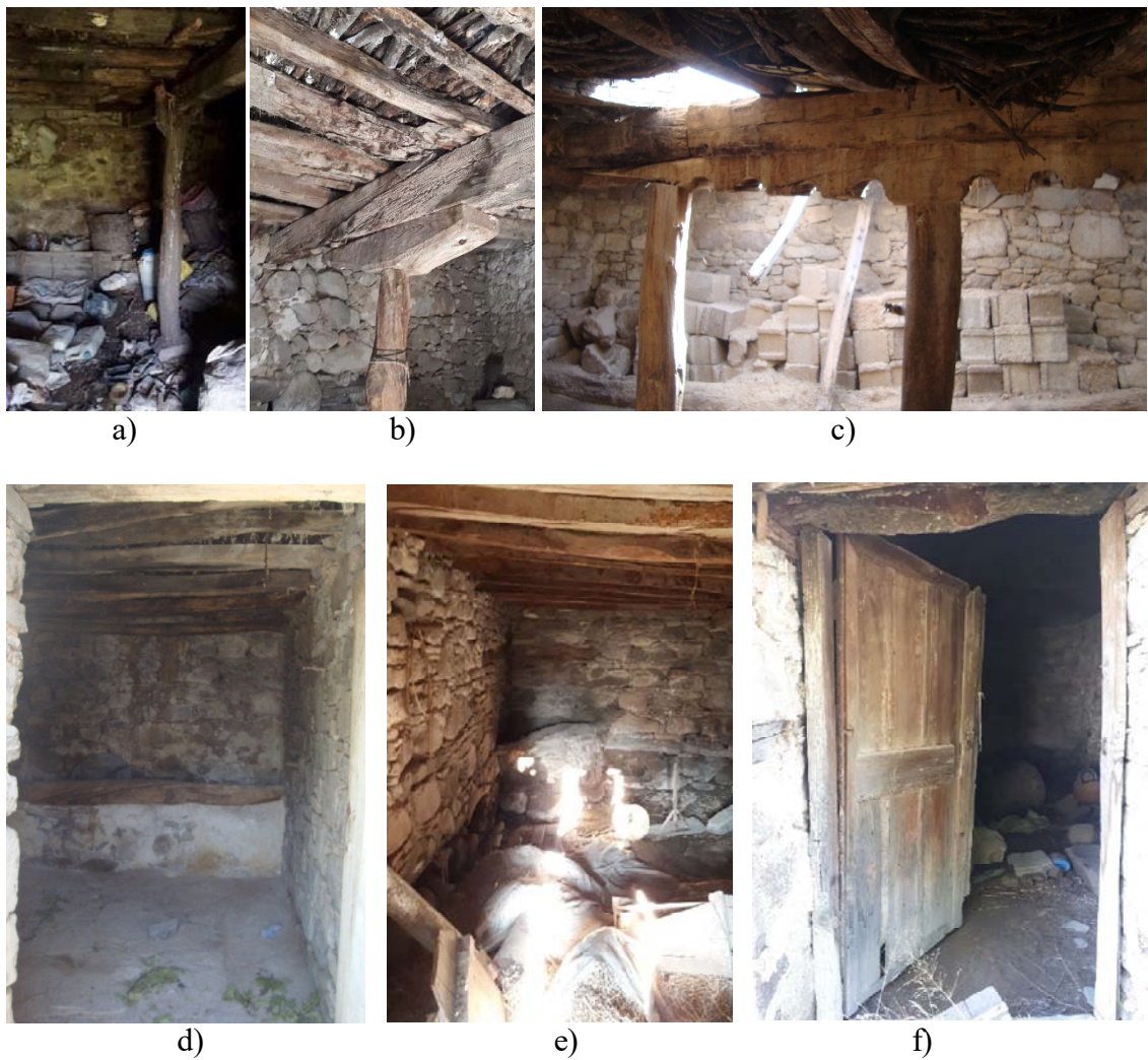
Figure 73. a) Padstone, Y shaped column. April 30, 2017. b) Column, transition element, main beam, joists, seren . April 26, 2017. c) Ornamented transition element. May, 2016. d) Slate stone ground covering, rectangular manger, wooden joists. May, 2016. E) Triangular manger at corner. April 24, 2017. f) Wooden door. April 24, 2017.
