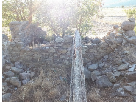
Dislocated main beam. September 24, 2017.
