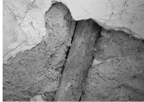
b) Deteriorated timber due to insect activity
