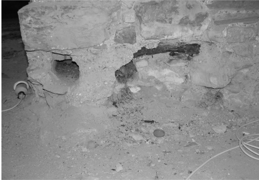
a) Deteriorated masonry wall ties, basement floor
