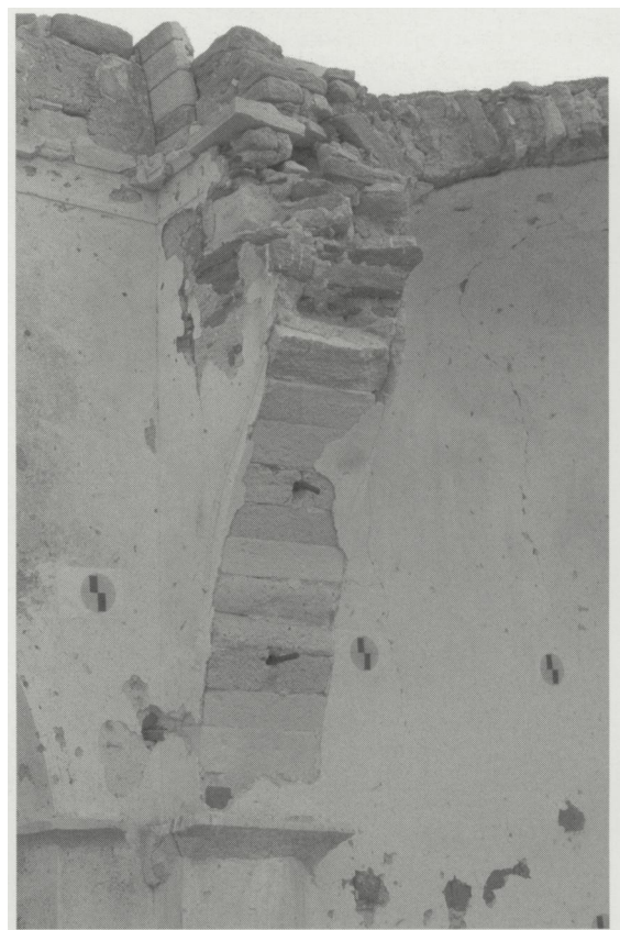
FIGURE 10. Photo illustrating the relation of the vault, arch, and pilaster on the southern part of the apse wall.
