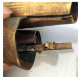
A stick entering the gap was welded to the other part. So that the two parts are connected to each other by these parts.
