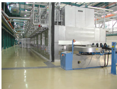
Figure 1 A view of the TD unit installed at Polinas Plastics Inc., Manisa, Turkey (see online version for colours)
