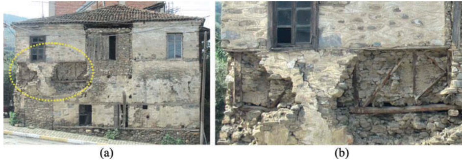
FIG. 7. (a) A damaged house built of double-leaf masonry; (b) close-up view of the outer stone masonry leaf and humuş inner frame (Kiraz-Yenişehir).
