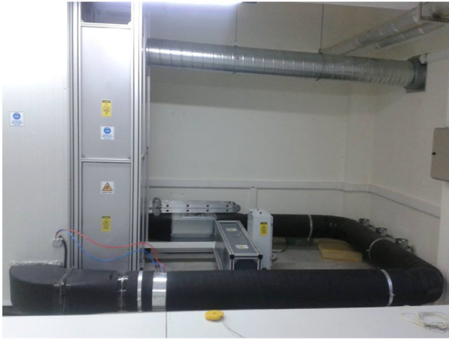
Fig. 3. General view of the duct system.
