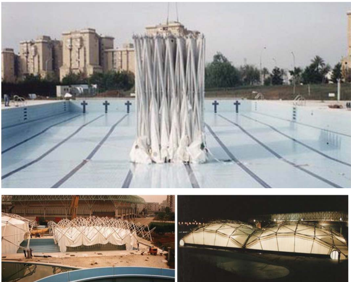
Figure 2.10. Deployable cover for a swimming pool in Seville designed by Escrig & Sanchez (Source: © Performance SL)
