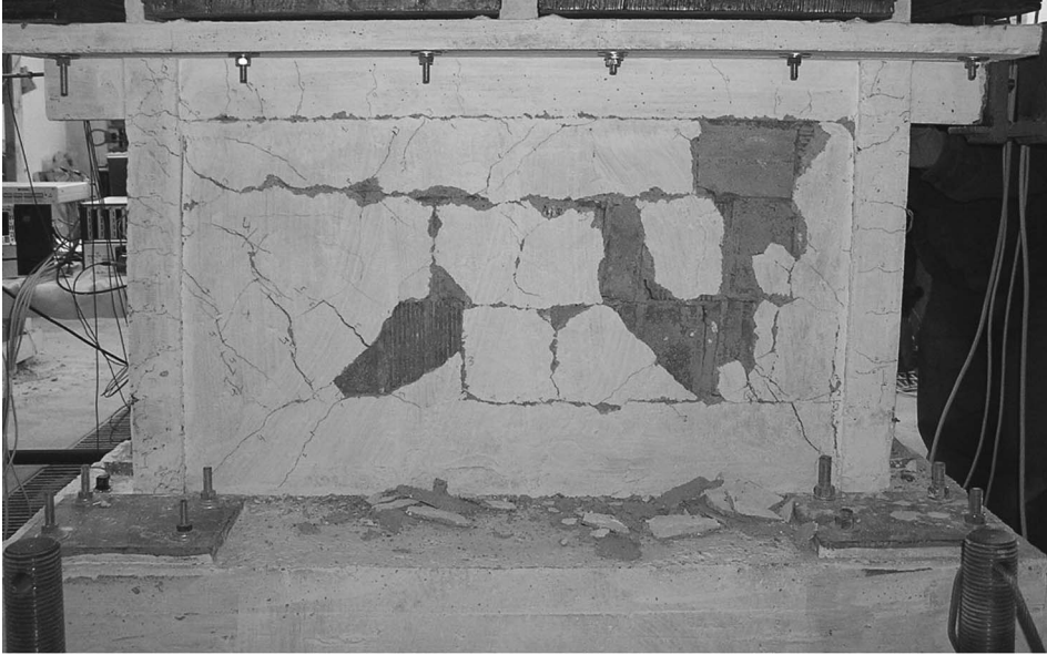
FIGURE 4 The damage in the 1 st story of Frame #3 after the 5 th loading group.
