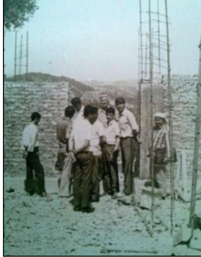
Figure 57. Collective Work in the Construction of Cooperative Olive Oil Factory (Source: Gödence Kooperatifi, 2016: 7)
