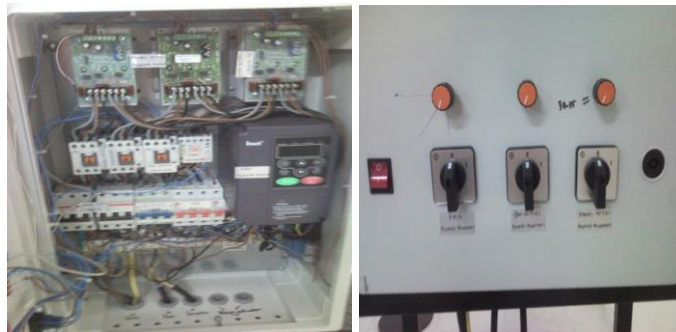
Figure 6.4. Control panel of fan and preheater
