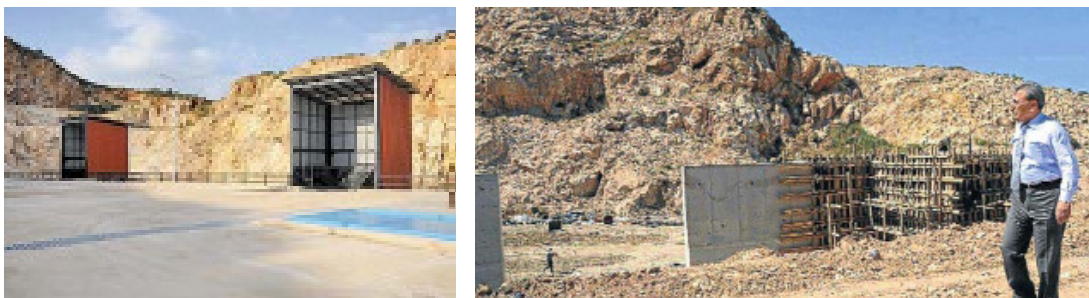
Figure 79. A quarry transferred to waste transfer station in Zeytinalanı (Source: left photo YA, 29.12.2010; right photo M, 30.12.2010)
