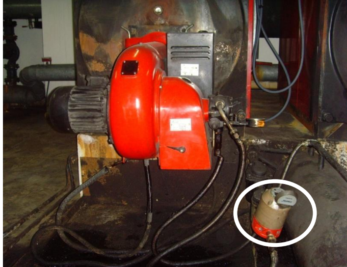
Figure 3.7. Flowmeter for boiler no:1.
