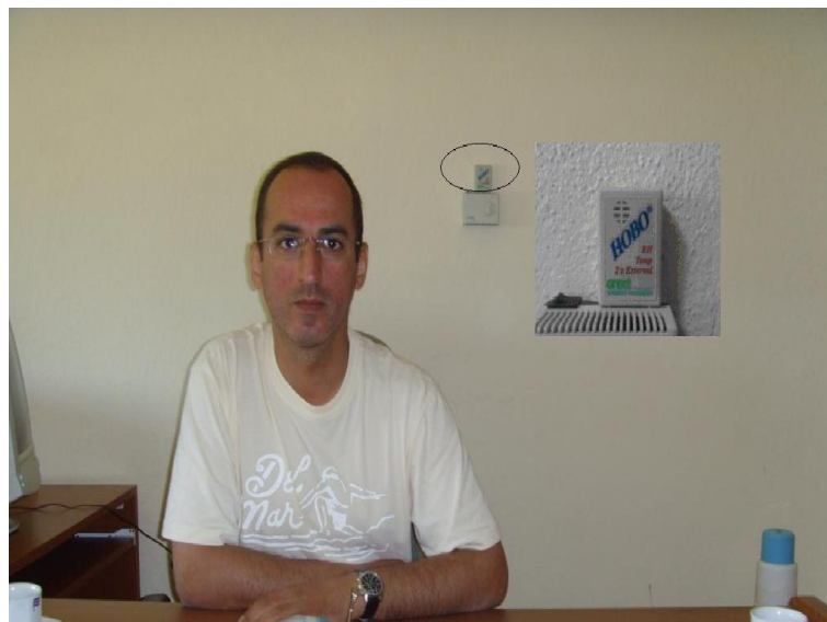
Figure 3.5. Datalogger installed in an office.
