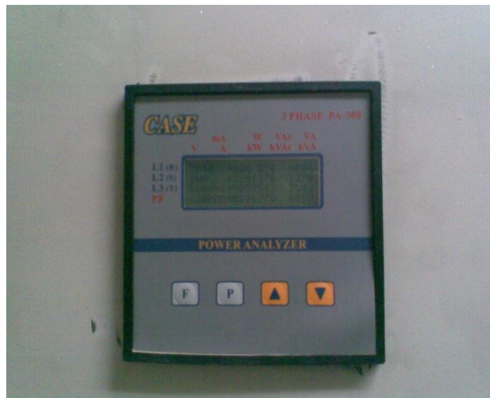
Figure 3.8. One of the power analyzers in the Administrative Building.
