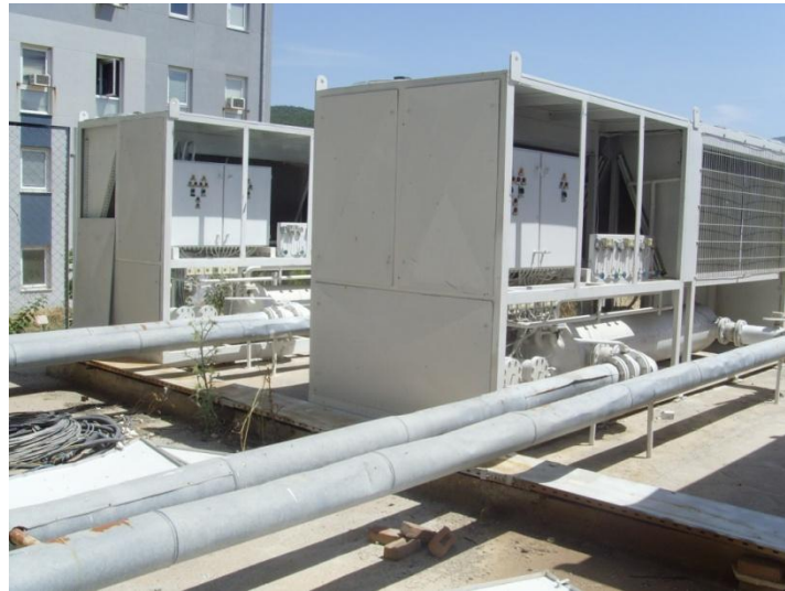
Figure 3.3. Cooling system of the the Administrative Building.
