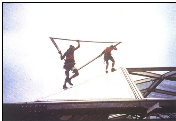
Fig.5.3. Workers Installing The Chelsea and Westminster Hospital Roof With a Part Of Frame Glazed with ETFE Source: AD 65, 1995
