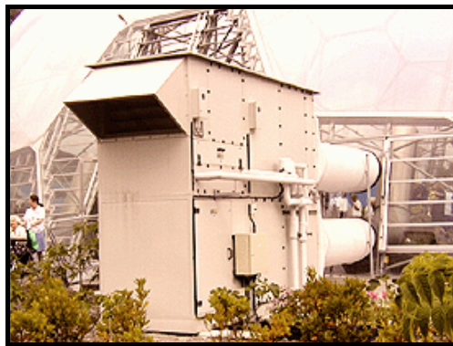
Fig. 3.18. Moducel LKS Air Handling Units provided by Eaton-Williams Co. Source: www.eaton-williams.com
