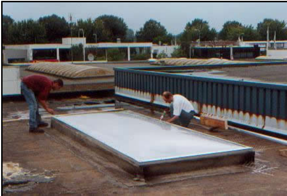
Fig. 3.53. Application Of IPS And Bird Protection String Around The Frame Source: www.buitink-technology .com
