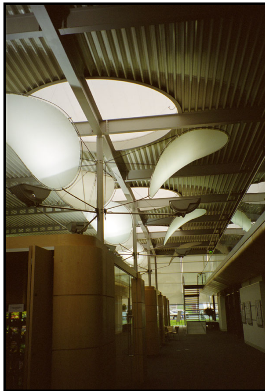
Fig. 3.45. Orange Company Light And Sound Wells And Rain Sound Suppressors
