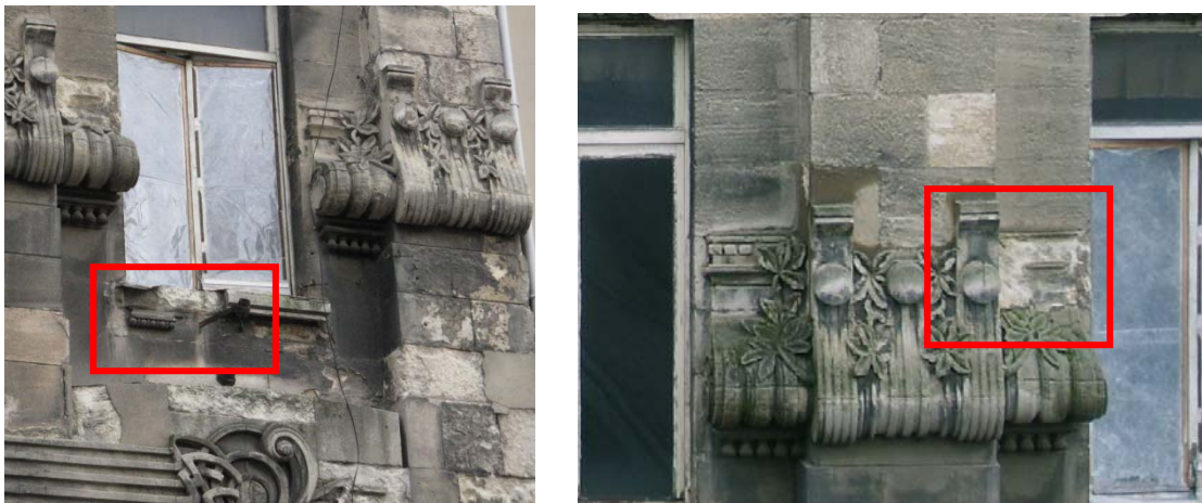
Figure 25. Break out on the façade of the Botter Apartment
