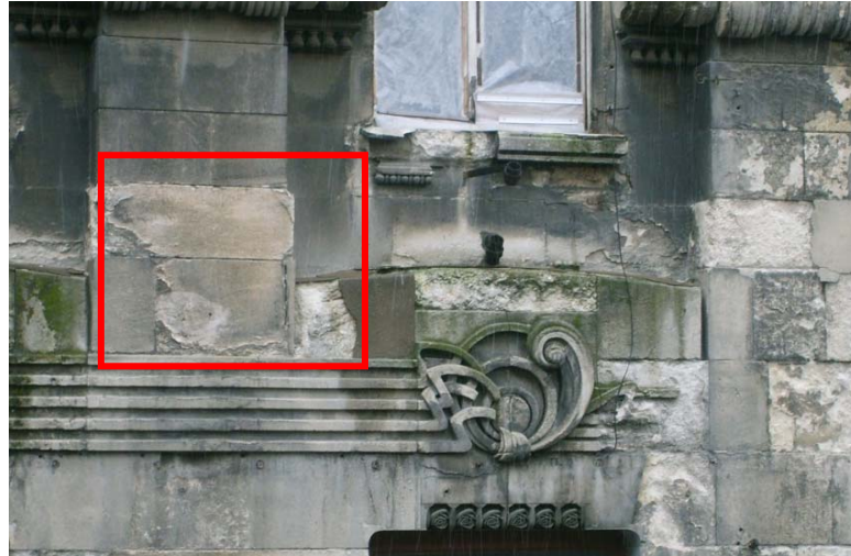
Figure 31. Scaling on the façade of the Botter Apartment
