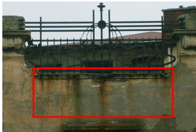
Figure 27. Coloration due to the corrosion products of the metals
