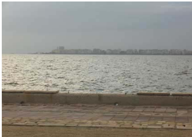
Figure 3.161. Broken Seating on the Parapet
