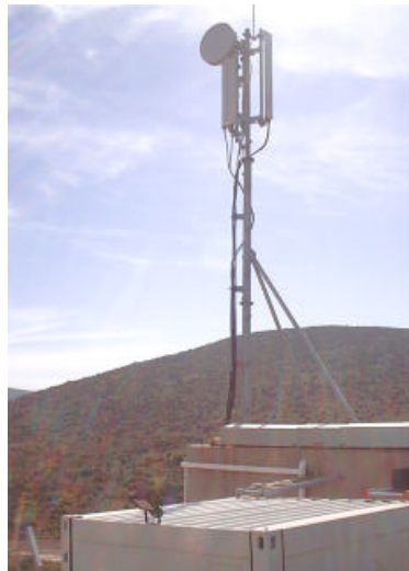
Figure 7.1 GSM base station
