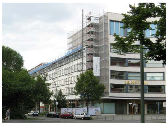
Figure 6.17. Erich Mendelshon, Metal Worker's Union Building , view from Lindenstraße, 1929 (Photography Feray Maden, August 2007)
