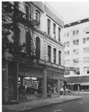
Figure 5.17. Thomas Mann Building – before vertical extension (Dibner A. and Dibner D. 1985, p.26)
