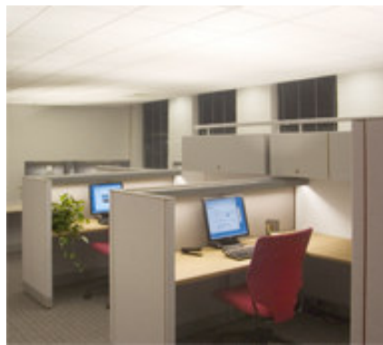
Figure 3.8. An Office with indirectly lighted ceiling. (Source: WEB_3 2005)
