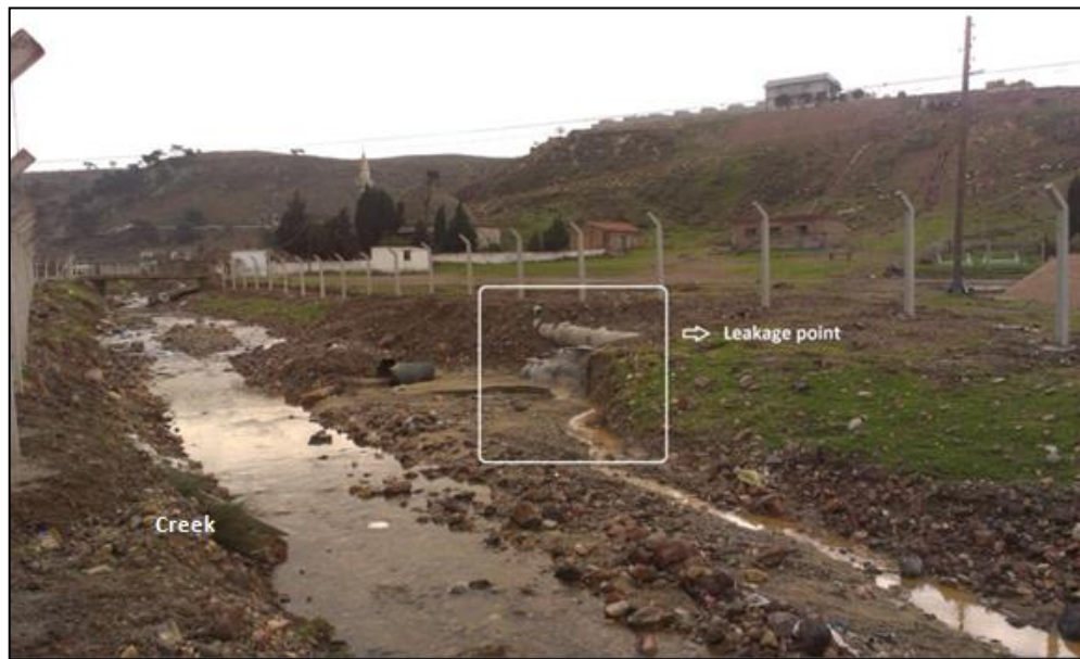
Figure 6.3. Leakage from Pipes and Discharge of Geothermal Fluid near The Creek
