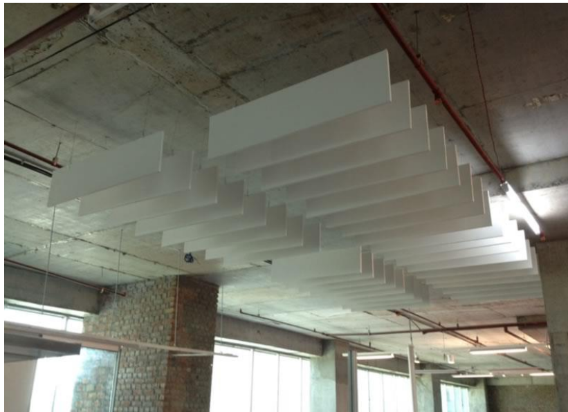
Figure 30. Acoustic baffles (Source: http://aktav.com.tr )
