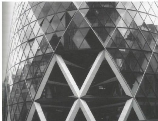
Figure 3. 36. Diagonal braced frame system, detail, 30 St. Mary Axe, London, UK, Foster and Partners (Source: Sandaker, Eggen, Cruvellier, 2011)
