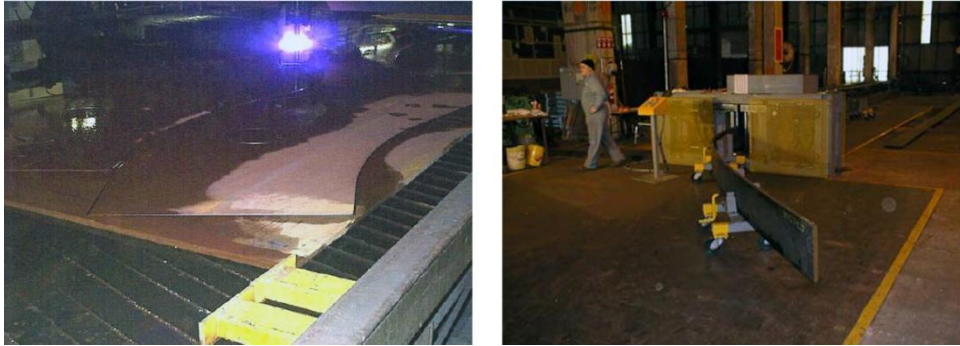
Figure 3. 64. Production process of I-sectioned frames, Experience Music Project, Frank Gehry (Source: Shelden, 2002)
