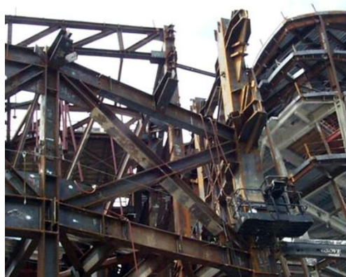
Figure 3. 33. Connection details of the braced frame system, Disney Concert Hall, Los Angeles, California, Frank Gehry (Source: Shelden, 2002)
