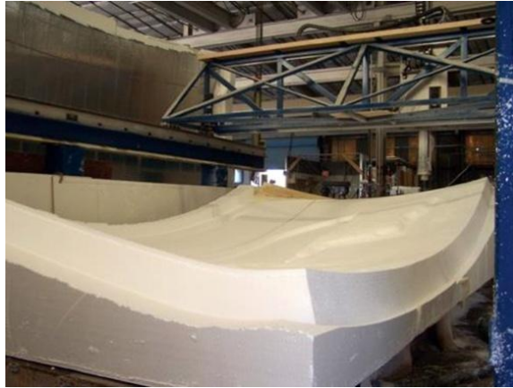
Figure 3. 71. CNC milling process of composite panels, California Bay House (Source: Composites Technology, 2010)
