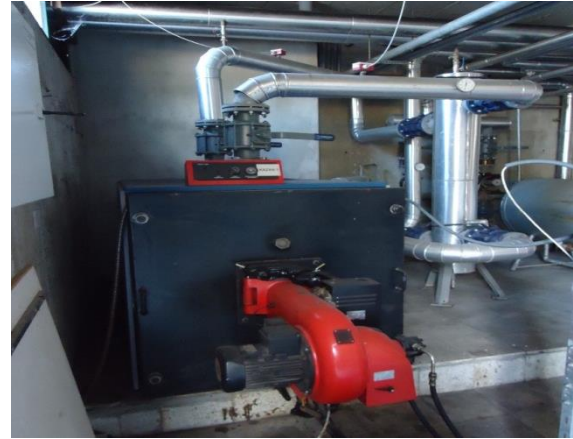
b.) Furnace System with Burner
