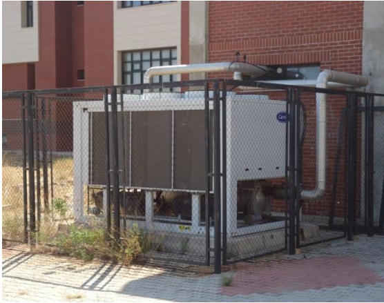
a.) Air to Water Chiller System
