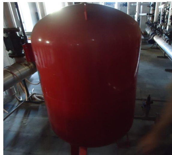
d.) Pressure Balance Tank
