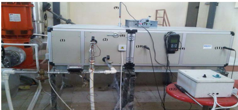
Figure 4.3. A view of geothermal drier
