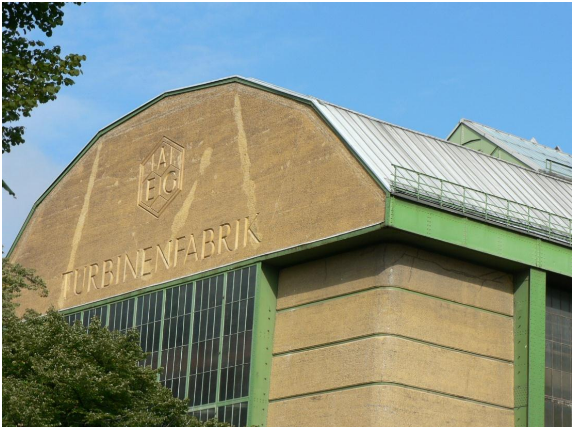
Figure 21. Turbine Factory Joint Detail of Gable, Pylon, Steel Pillars and Lintel (Source: Photo by Author)
