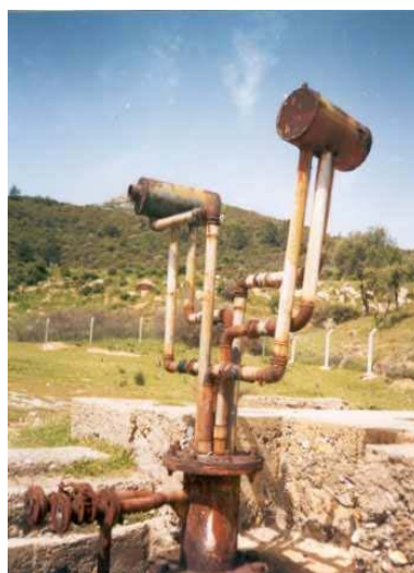
Fig 2.2 Downhole heat exchanger system (Seferihisar,İzmir)
