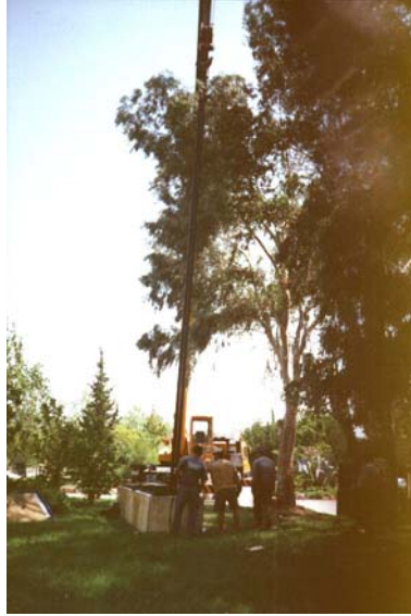
Fig 2.1 Downhole heat exchangers being removed from a well in Balçova (3-8-2001)
