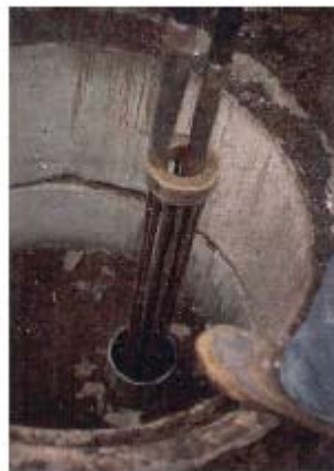
Fig 1.3 Test project using multiple loops being lowered in a well (Klamath Falls) [8].
