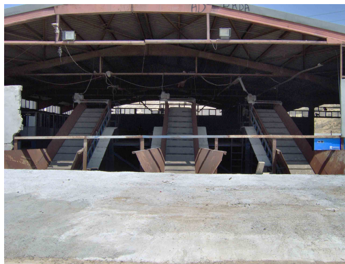
Figure 3.14 Three number manual sorting lines of Harmandalı sorting facility
