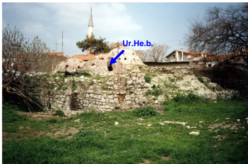
Figure 3.14 View from the southeast elevation of the Hersekzade Bath in Urla, showing where brick masonry mortar samples (Ur.He.b.) were collected.
