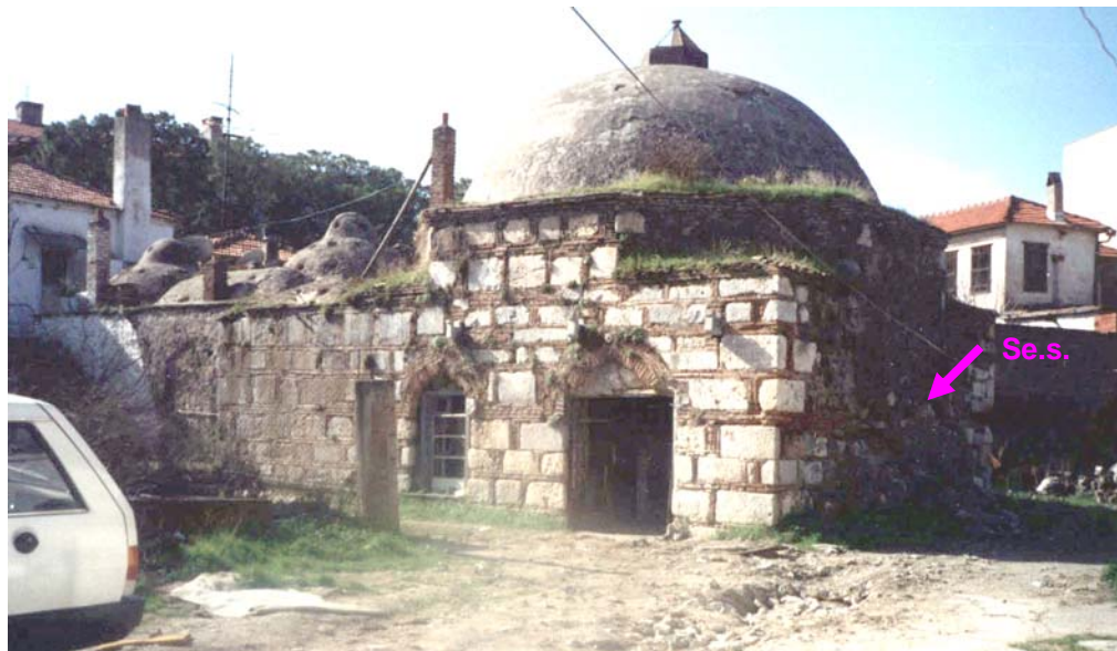
Figure 3.2 View from the east and north elevations of the Seferihisar Bath, showing where stone masonry mortar samples (Se.s.) were collected.
