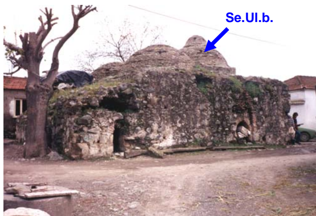
Figure 3.9 View from the northwest elevation of the Ulamiş Bath in Seferihisar, showing where brick masonry mortar samples (Se.Ul.b.) were collected.
