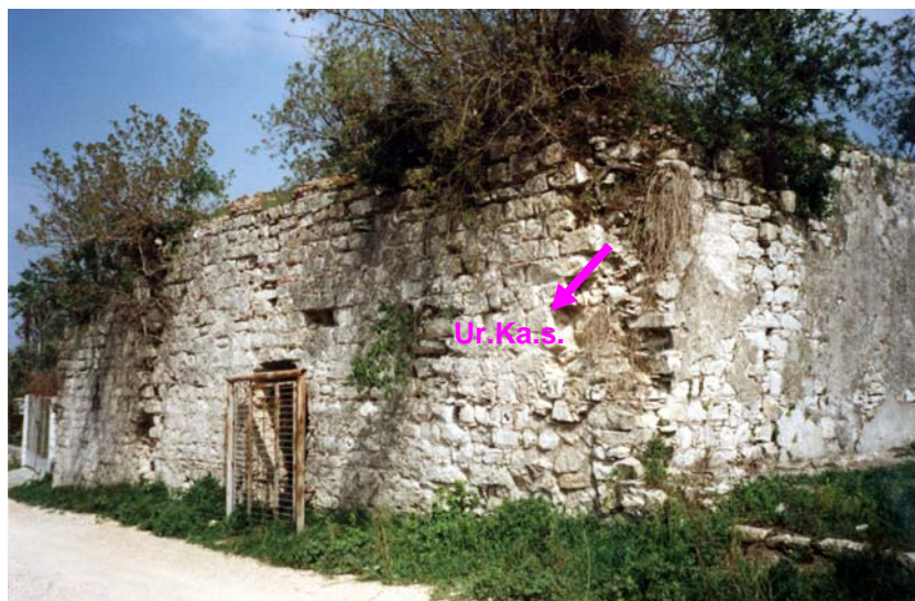
Figure 3.16 View from the northwest elevation of the Kamanlı Bath in Urla, showing where stone masonry mortar samples (Ur.Ka.s) were collected.
