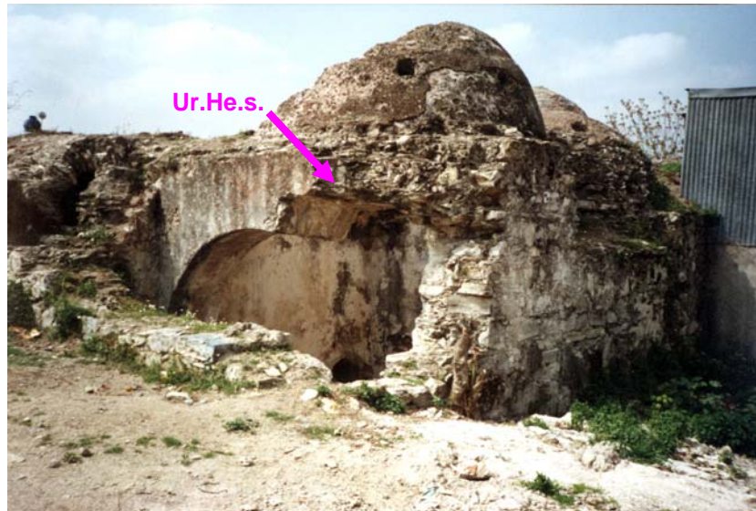
Figure 3.13 View from the southeast elevation of the Hersekzade Bath in Urla, showing where stone masonry mortar samples (Ur.He.s.) were collected.
