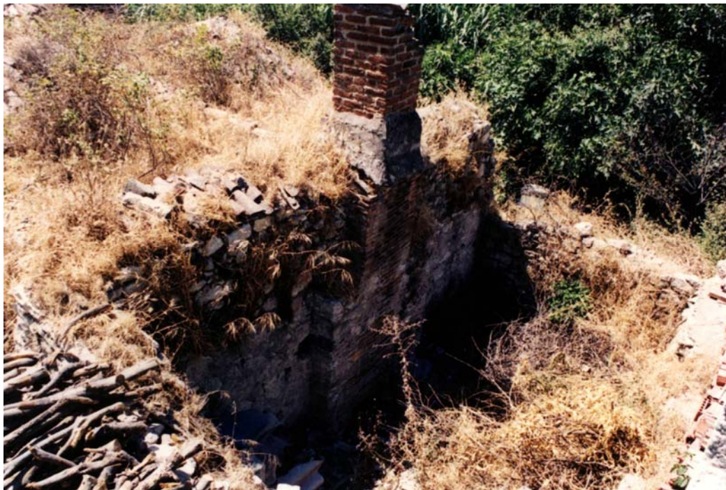
Figure 3.71. Urla Özbek Hamam, The Furnace
