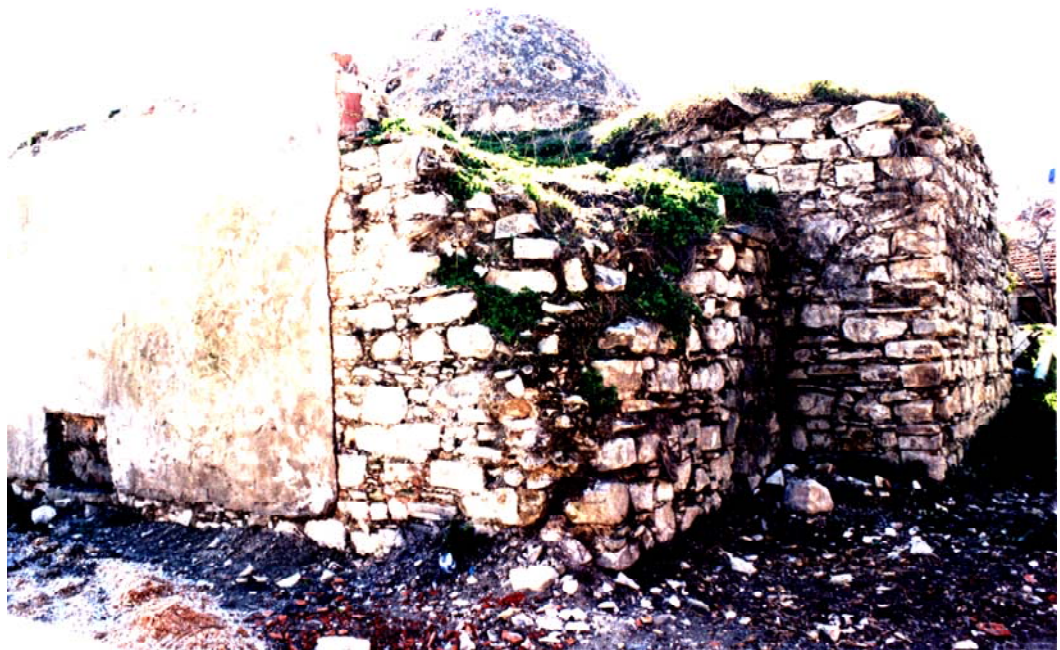
Figure 3.43. Urla Çifte Hamam, The Northwest Facade, Rubble Stone Bond of the Exterior Walls
