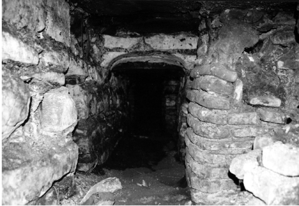
Figure 3.46. Urla Çifte Hamam, The Use of Stone Lintel above the opening of the Masonry Walls in the Cehennemlik Section
