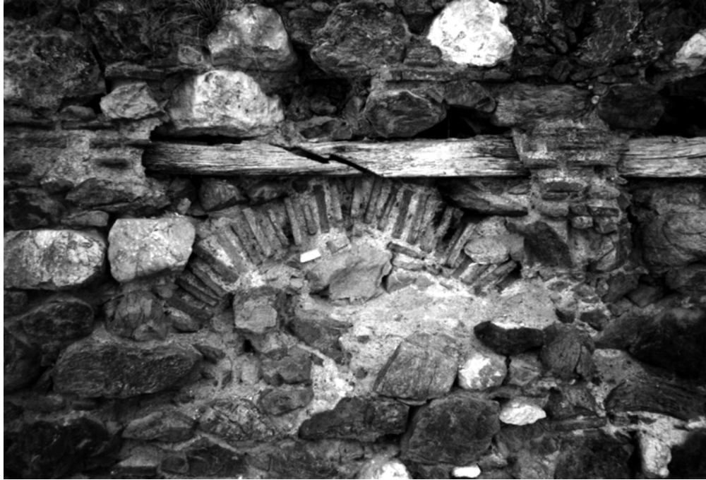
Figure 3.23. Seferihisar Büyük Hamam, The Use of Timber Beam in the Exterior North Wall.
