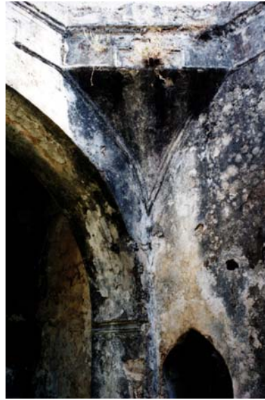
Figure 4.15. Urla Çifte Hamam, Pendentive in the Main Sıcaklık Space of the Men' s Section
