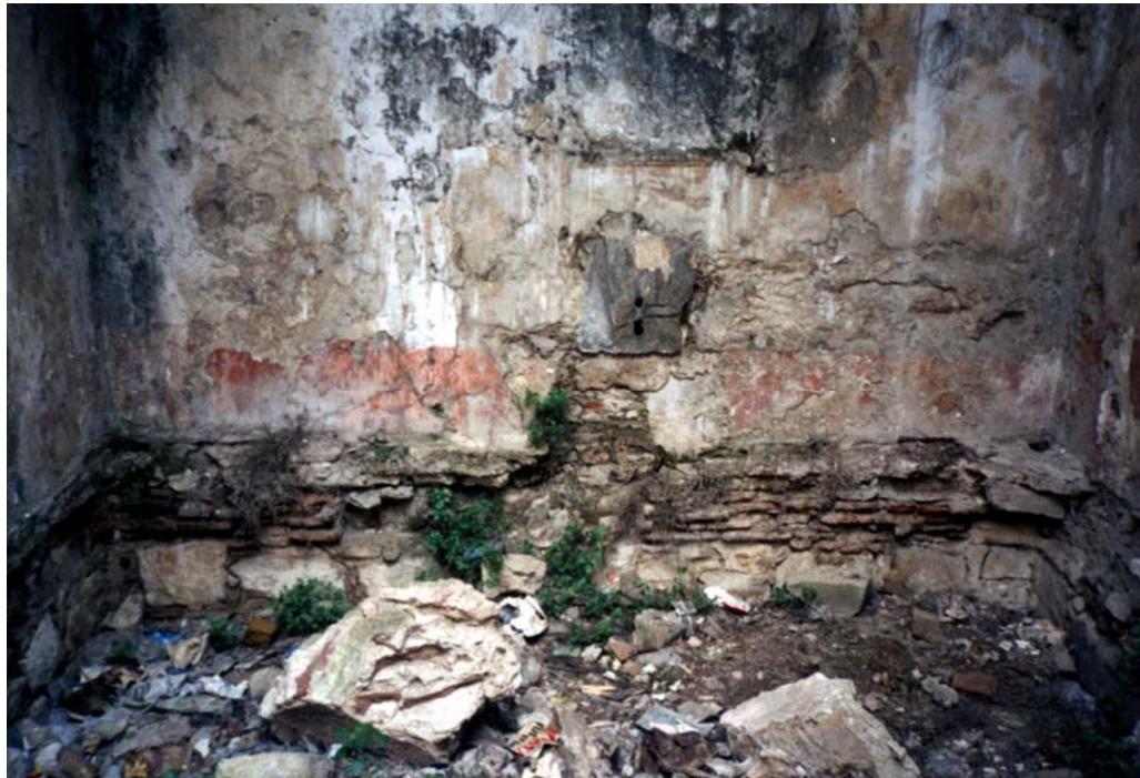
Figure 3.47. Urla Çifte Hamam, The Use of Tap Panel on the Walls in the Main Sıcaklık Space of Men's Section
