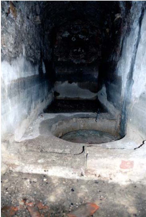
Figure 3.70. Urla Özbek Hamam, The Use of Water Boiler in the Water Reservoir
