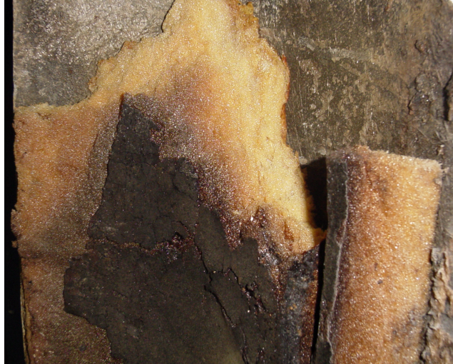
Figure 4.4. Deformation of polyurethane insulation in Balçova-Narlıdere GDHS.
