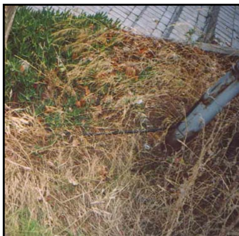
Figure 4.18 The exposed overground cables
