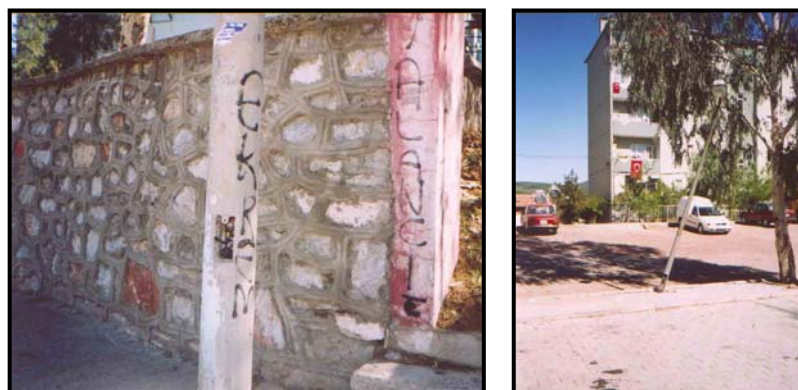
Figure 4.25. The existing fixtures damaged
