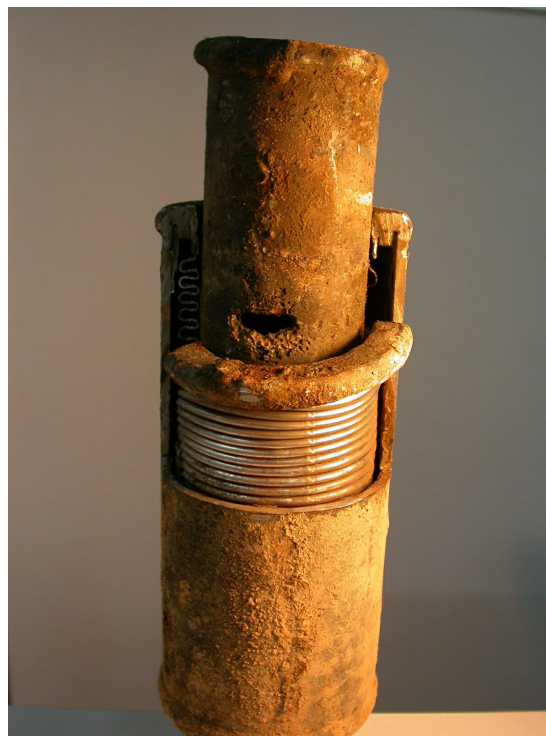
Figure 2.15. Corrosion caused by the galvanic effect on a compensators taken from Balçova-Izmir geothermal system.
