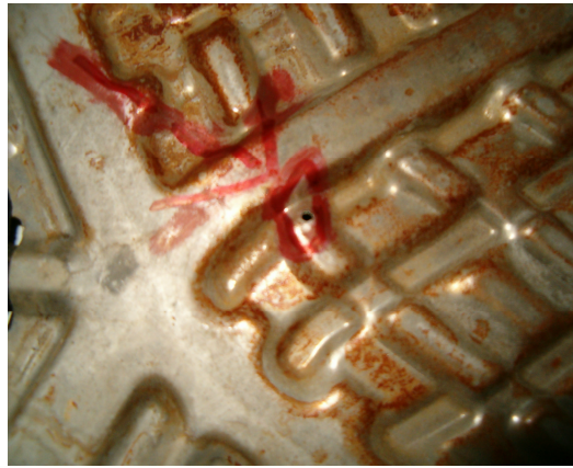
Figure 2.12. Pits on the surface of a stainless heat exchanger.
