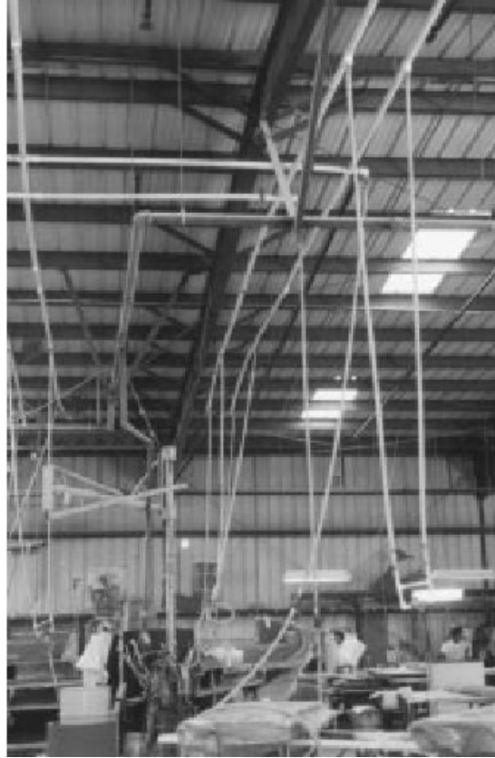
Figure 4.31. Overhead High- and Low-Pressure Vacuum Lines. (Greene 2004)
