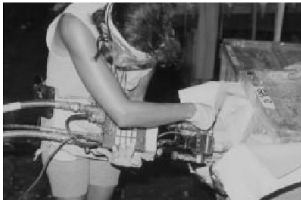
Figure 4.46. Two-Part Expansion Foam is Injected into Stringer Molds at Compsys with Careful Monitoring of Material Flow rate and Duration (Greene 2004)
