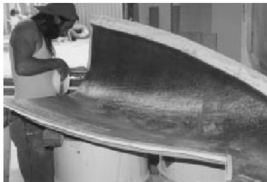
Figure 4.30. Sealing Tape is applied to Mold Prior to Vacuum Bag Use (Greene 2004)
