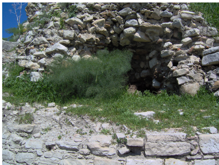
Figure 4.22. Loss of intact stone blocks
