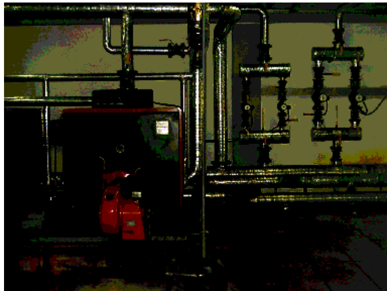
Figure 2.2: A view of the Heat centre in the Faculty of Engineering
