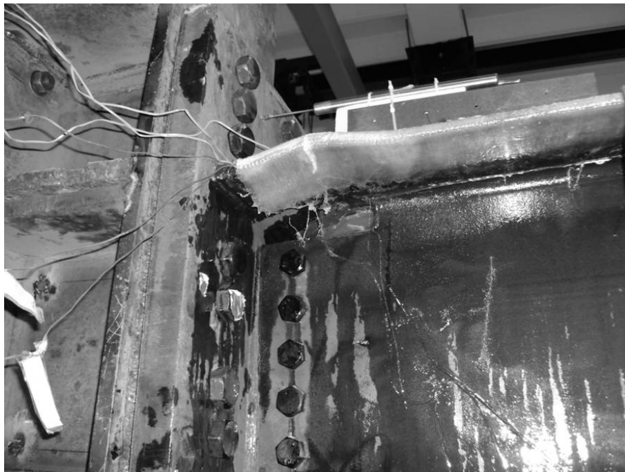
Figure 4.28. HE500AA GFRP1 Beam Top Flange at 0.033 rad of Rotation
