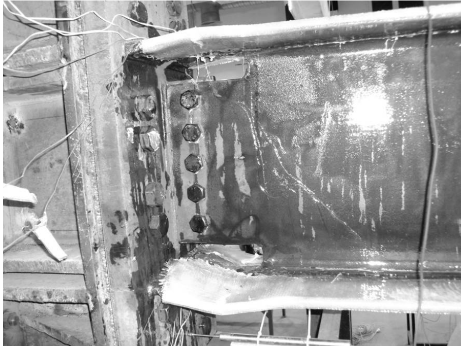
Figure 4.29. HE500AA GFRP1 Beam GFRP Debonding at 0.036 rad of Rotation
