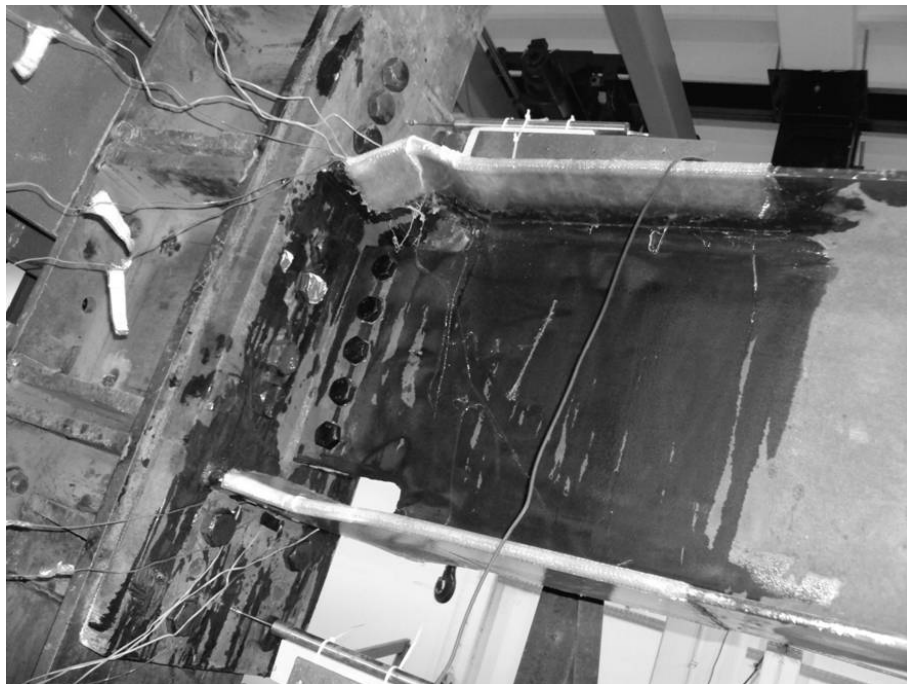
Figure 4.30. HE500AA GFRP1 Beam Top Flange at 0.043 rad of Rotation
