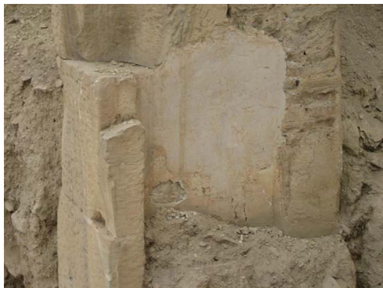
Figure 3. 7. Loss of plaster layers on the wall.
