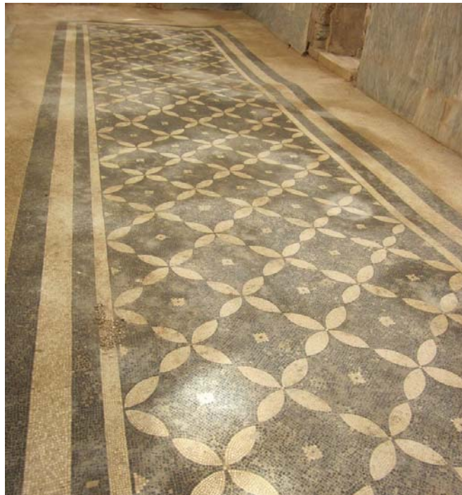
Figure 3. 2. Wetting of the mosaics due to rising damp.
