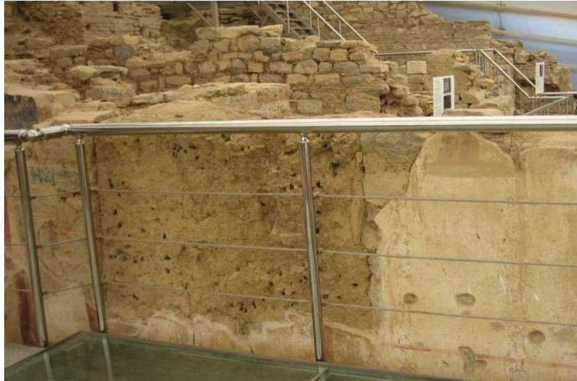
Figure 4. 1. Cavities in the wall structure at the Terrace House 2 at Ephesus (Turkey).
