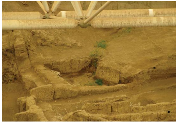
Figure 3. 8. Plants due to lack of roof and site drainage at south shelter.
