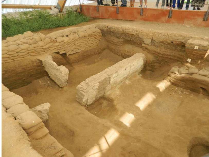
Figure 3. 10. Basal erosion and presence of plants due to rising damp at north shelter.
