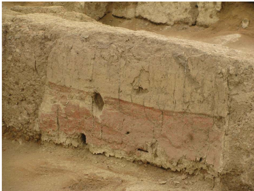
Figure 3. 11. Loss of plaster layers at the north shelter.
