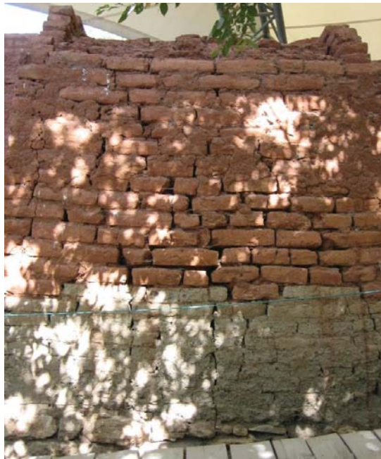
Figure 3. 14. Loss of mud mortar and structural cracks on the reconstructed fortification wall at the Citadel Wall and the Megaron at Troy (Turkey).
