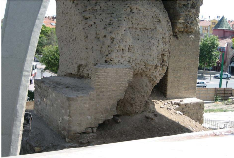
Figure 3. 12. Basal erosion due to rising damp.
