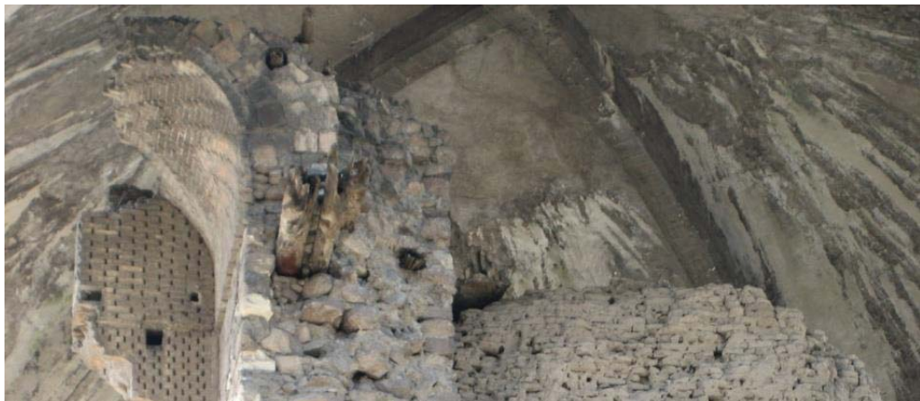
Figure 4. 3. Percolation through cracks in the roof material.
