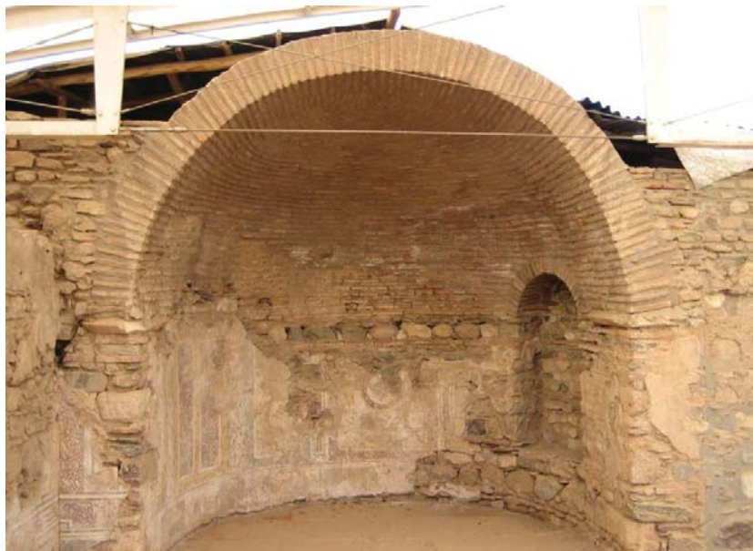
Figure 3. 5. Salt crystallization due to limited shelter area.
