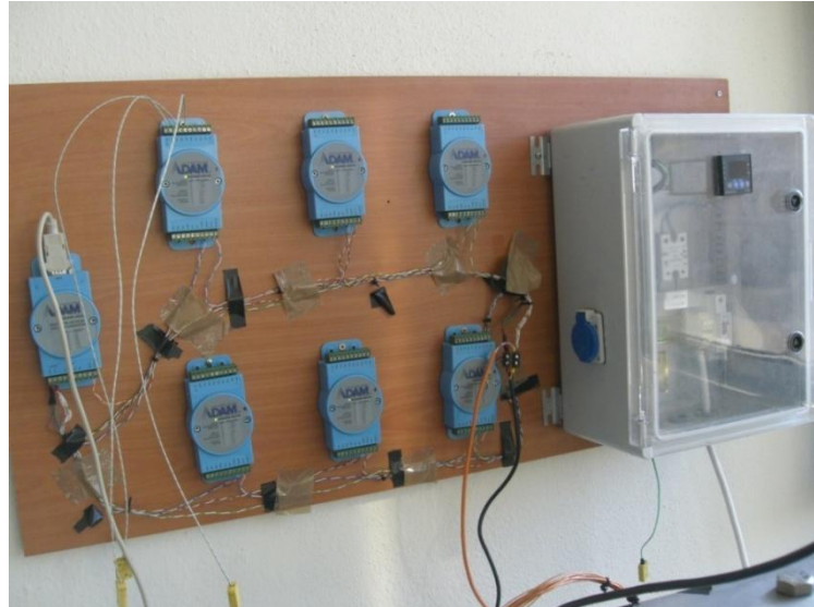
Figure 7.3. Data logger set and the electrical resistance control panel
