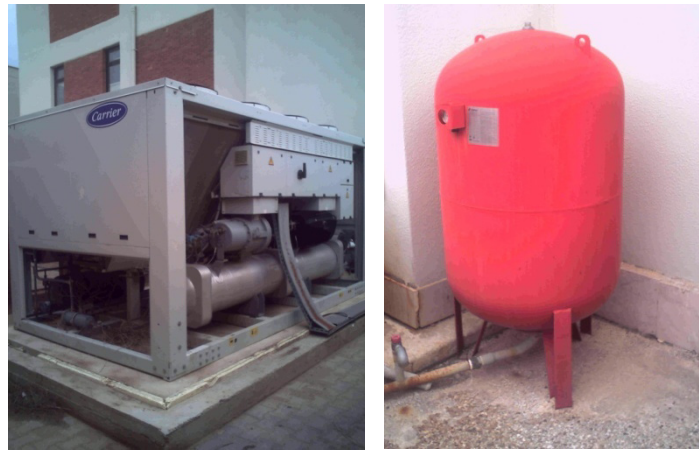
Figure 35. Chiller and condenser of the cooling installation
