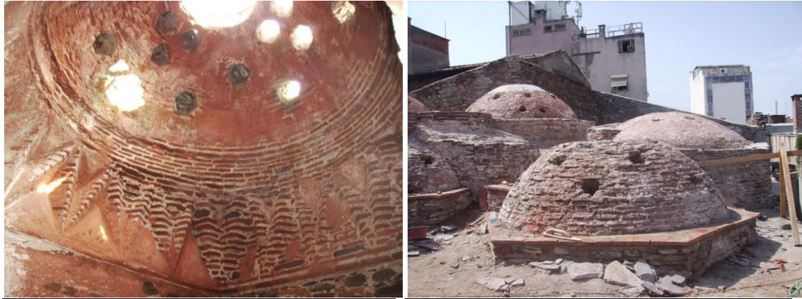
Figure A.10. Tire Tahtakale Hamami, interior and exterior views of northeast halvet dome.
