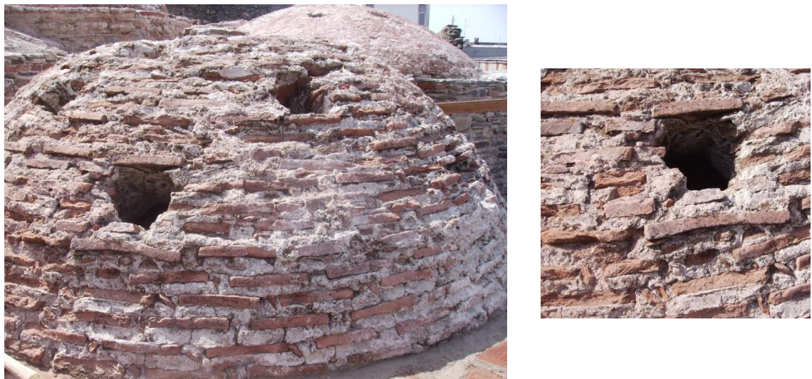
Figure 3.29. In Tire Tahtakale Hamami men’s section northeast halvet dome using the bond type of “ random horizontal stacking of long and short faces ”.
