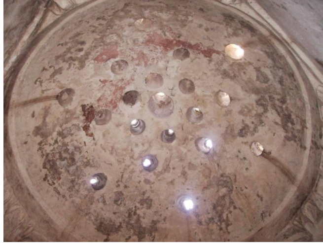
Figure A.28. Tire Mehmet Ağa Hamamı women's section, interior view of sıcaklık main space dome.
