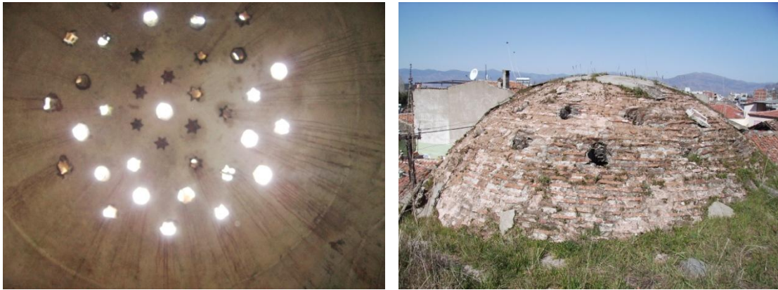
Figure A.44. Tire Yalınayak Hamamı men's section, interior and exterior views of the north corner halvet dome.
