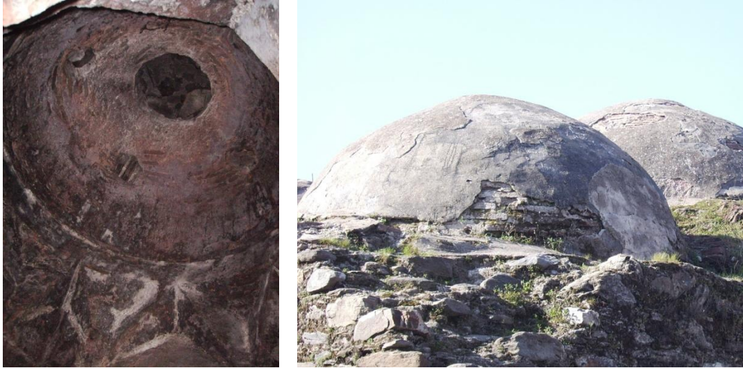
Figure A.48. Tire Yeniceköy Hamamı, interior and exterior views of southeast İliklik sub-unit dome.
