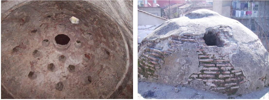
Figure A.51. Tire Yeniceköy Hamamı, interior and exterior views of southwest halvet dome.
