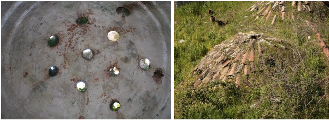
Figure A.103. Özbek Köyü Hamamı, interior and exterior views of northeast halvet dome.
