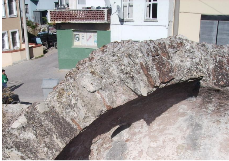
Figure 3.33. In the dome of Urla Hersekzade Ahmet Paşa Hamamı men's section ılıklik space using the irregular brick / stone bond.
