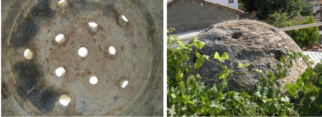
Figure A.79. Sığacık Kaleiçi Hamam, interior and exterior views of southwest halvet dome.
