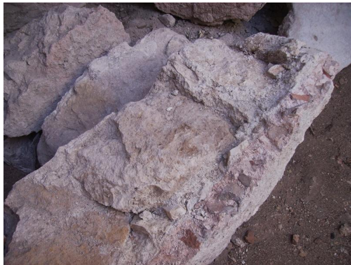
Figure 3.35. A part of collapsed dome in Urla Hersekzade Ahmet Paşa Hamamı men’s section sıcaklık main space. “ irregular stone bond formed by random and irregular stacking of rubble and cut stone ” with horasan coating composed of large and small pieces of brick can be seen on the figure.
