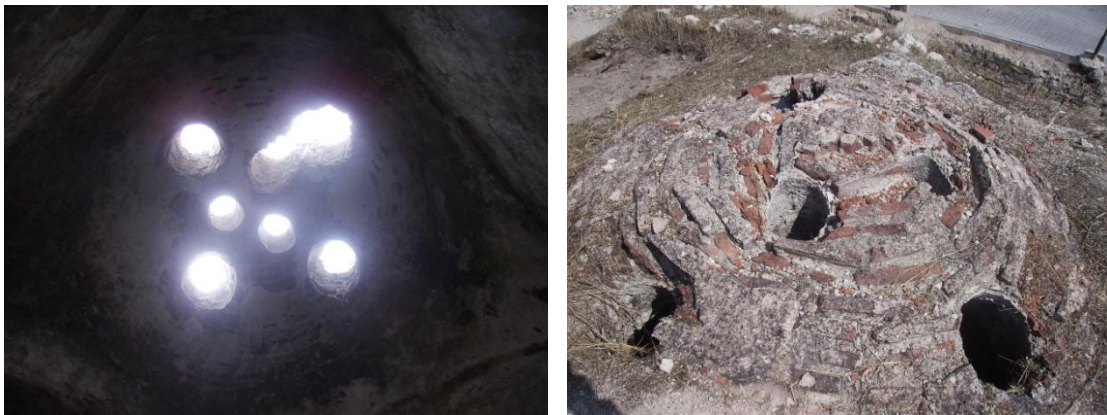
Figure A.84. Urla Hersekzade Ahmet Paşa Hamamı, interior and exterior views of İliklik dome in the women's section.
